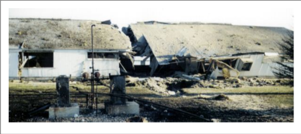
Fig. A.1. Structural damage from BLEVE blast and fragment impact (Source: US CSB www.csb.gov )
