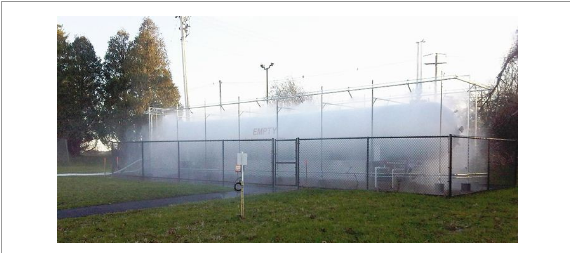
Fig. 9. Water spray discharge on a 15,000 gal (58 m 3 ) LPG tank (FM SimZone)
