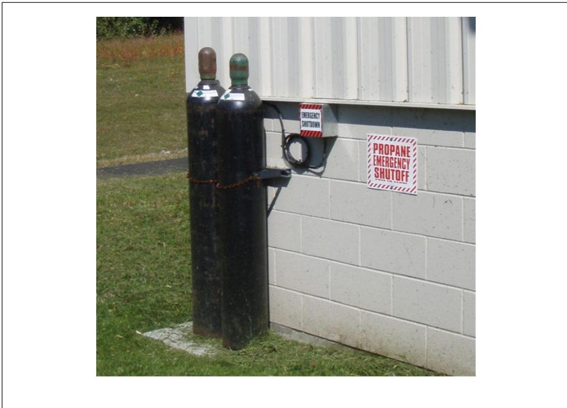
Fig. 10. Remote emergency shutoff 75 ft (23 m) from LPG tank (FM SimZone)
