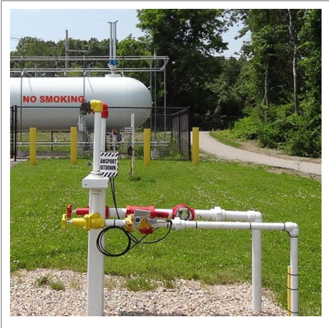
Fig. 7. LPG unloading station 50 ft (15 m) away from storage tank (FM SimZone)
