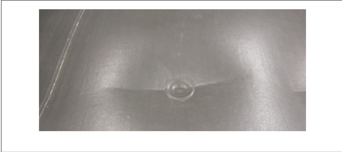
Fig. D.4.2.2-2. Crease in single-ply roof cover while subjected to uplift pressure
