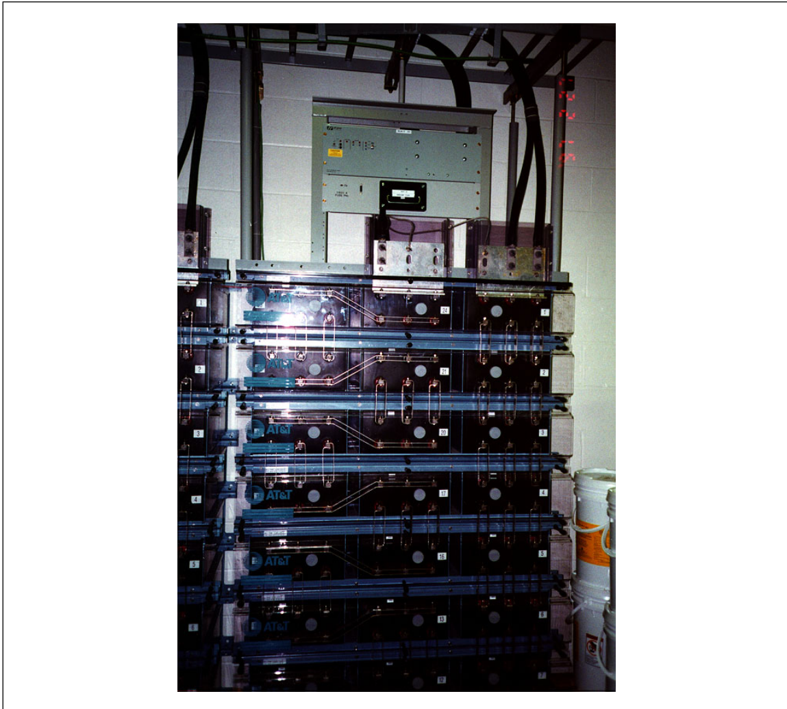
Fig. 10. Valve-regulated lead acid batteries
