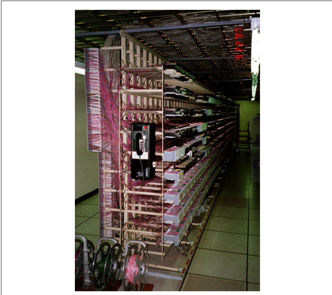
Fig. 8. Main distribution frame (MDF)
