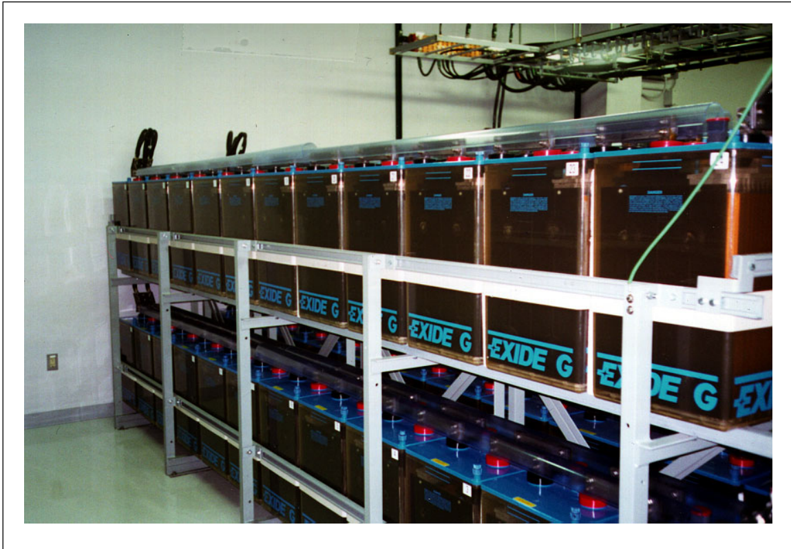
Fig. 9. Flooded-cell battery room
