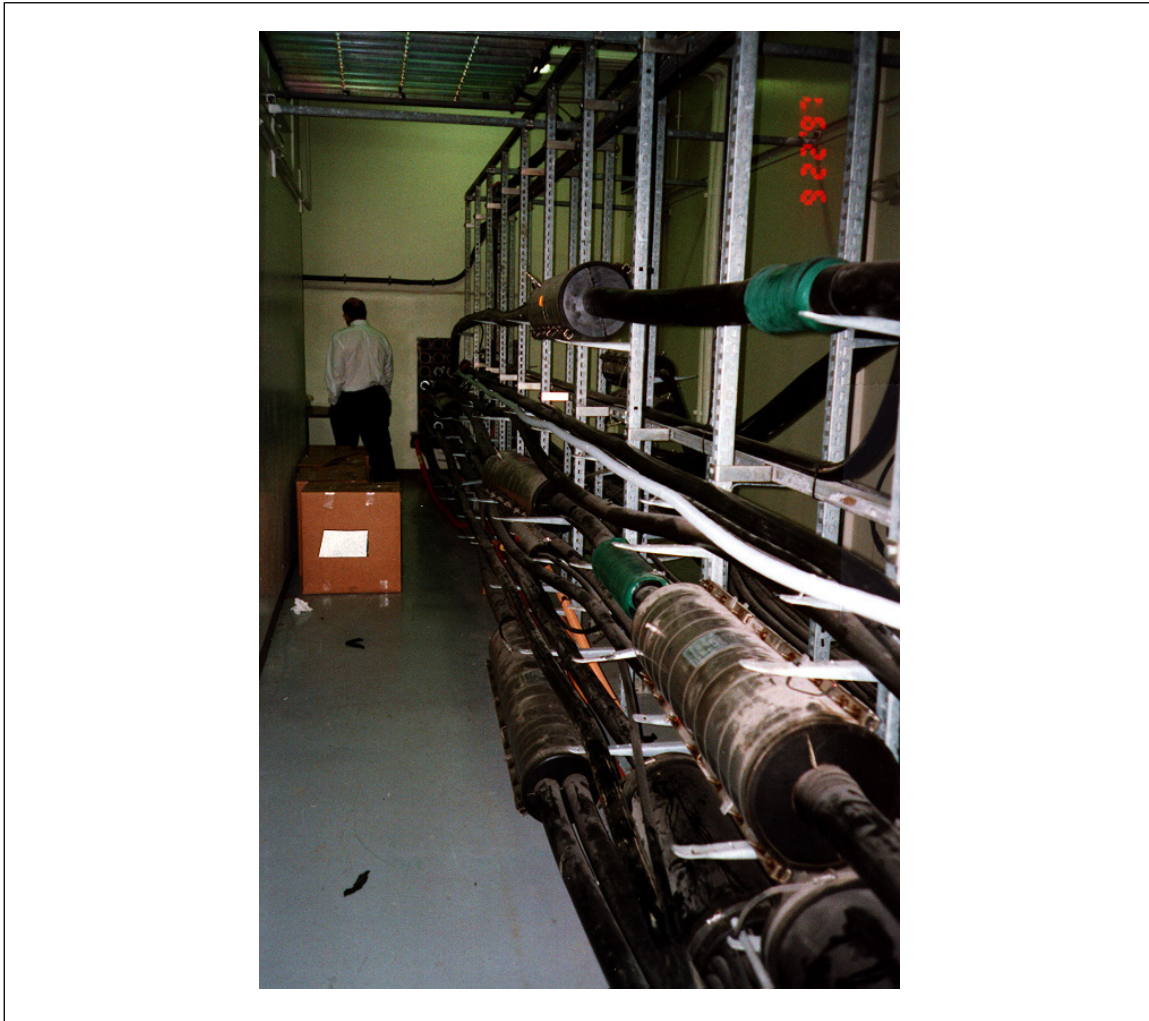
Fig. 6. Cable tunnel for an end office
