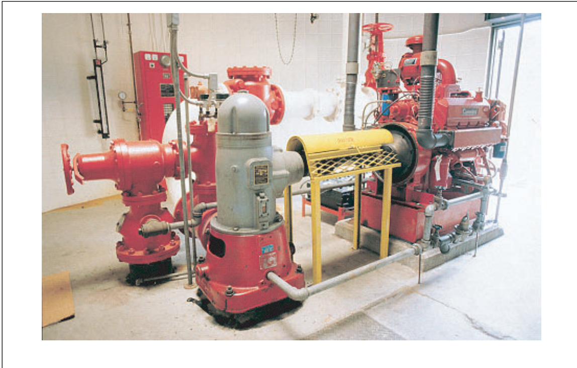
Fig. 2.2.1.2-1 Photo of well arranged pump room
