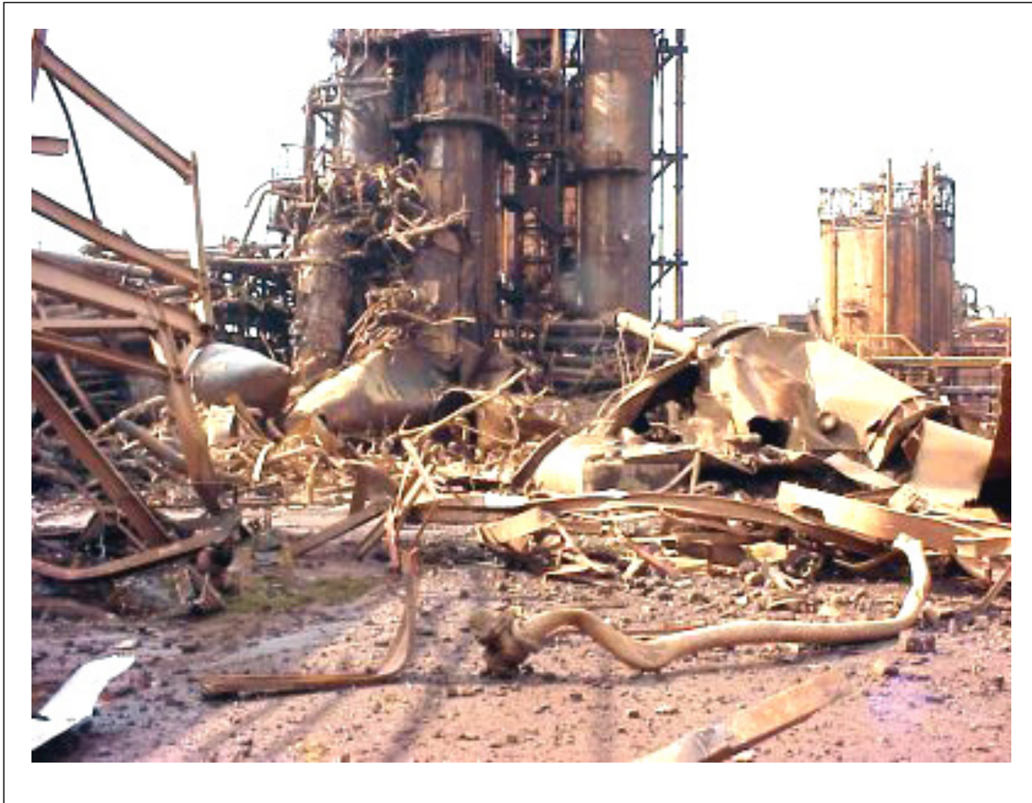
Fig. 2. Damage after the explosion.
