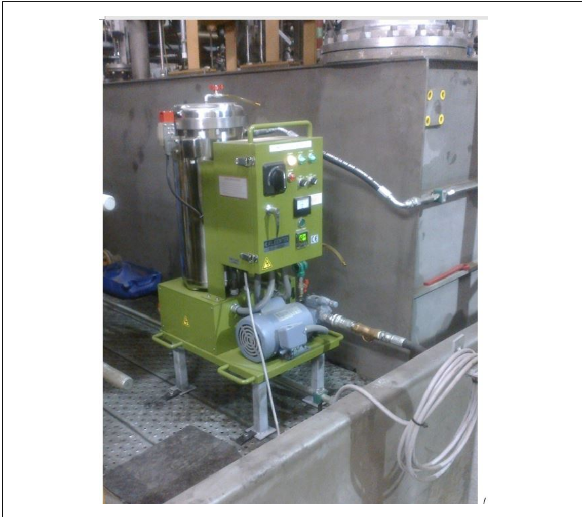
Fig. 2.2.5.4.1. Lube oil purifying skid inside containment area
