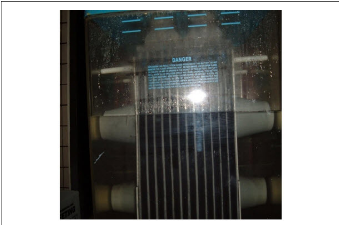
Fig. 3. Severely low electrolyte observed at visual inspection
