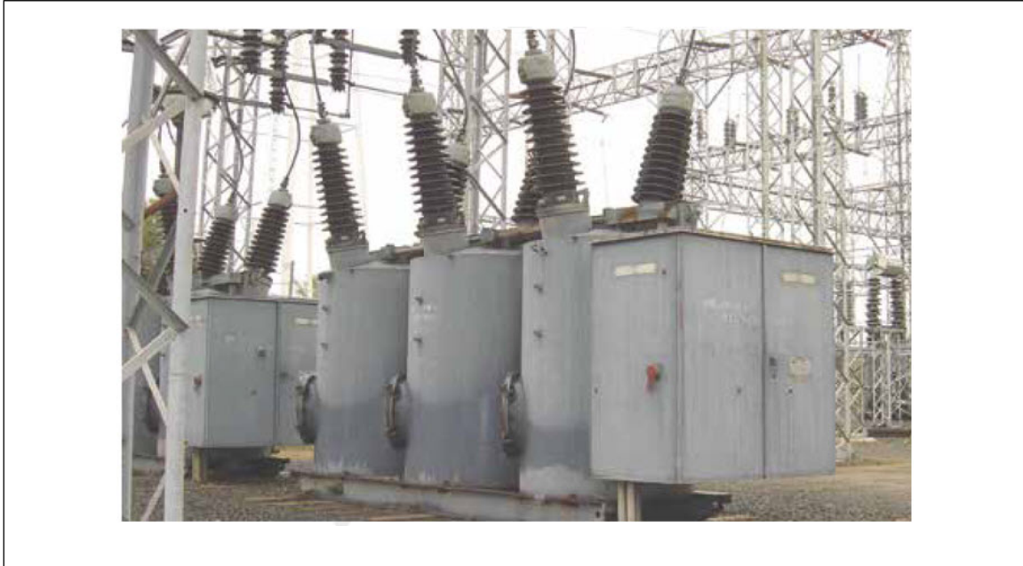
Fig. 5. Bulk Oil circuit breaker
