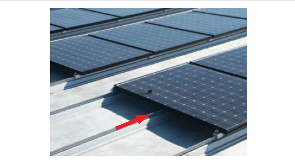
Fig. 3.2.2b. Unacceptable arrangement unless specifically tested and FM Approved: clamp missing from SSR rib below middle of outer panel edge
