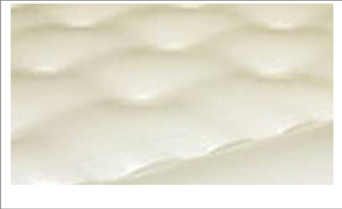
Fig. 3.2.1.1a. Mechanically fastened roof cover billowing when subjected to wind pressure
