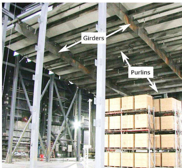
Figure 2-22: Ceiling structure for Test #5 showing 460 mm (18 in.) purlins and 610 mm (24 in.) girders attached to the flat part of the ceiling. Purlin channels at girders are closed.
