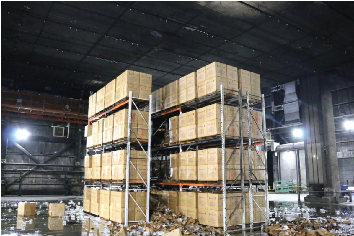
Figure E-5: Baseline post-test photograph of the east face of the main array showing fire damage.
