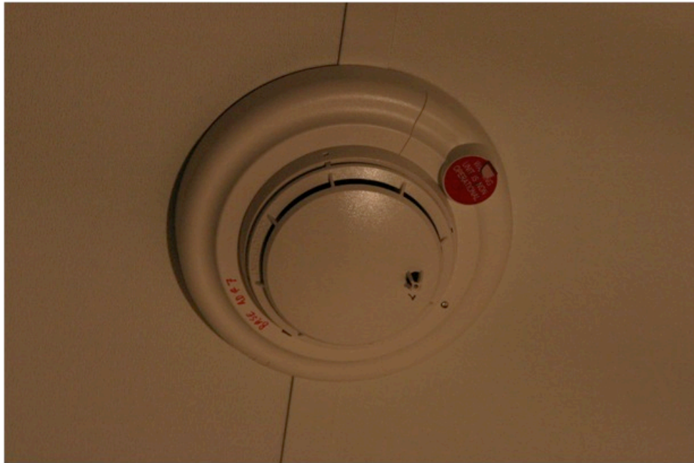
Figure 2-22: Combination photoelectric smoke detector (Spot-S)
