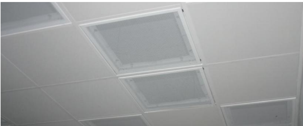
Figure 2-11: Photograph of ventilation return grates in the suspended ceiling.
