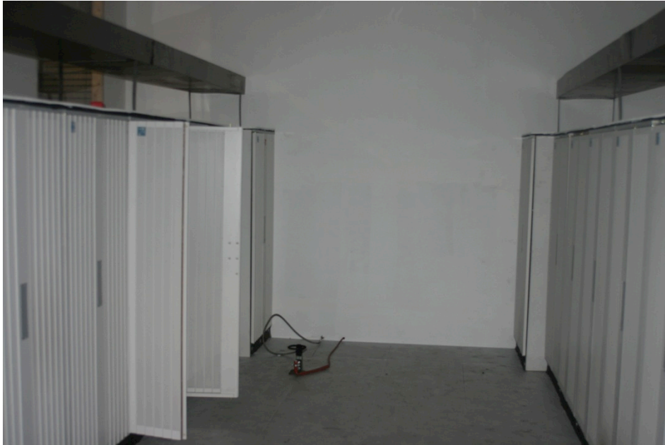
Figure 2-14: Picture showing the server cabinets in the hot aisle.
