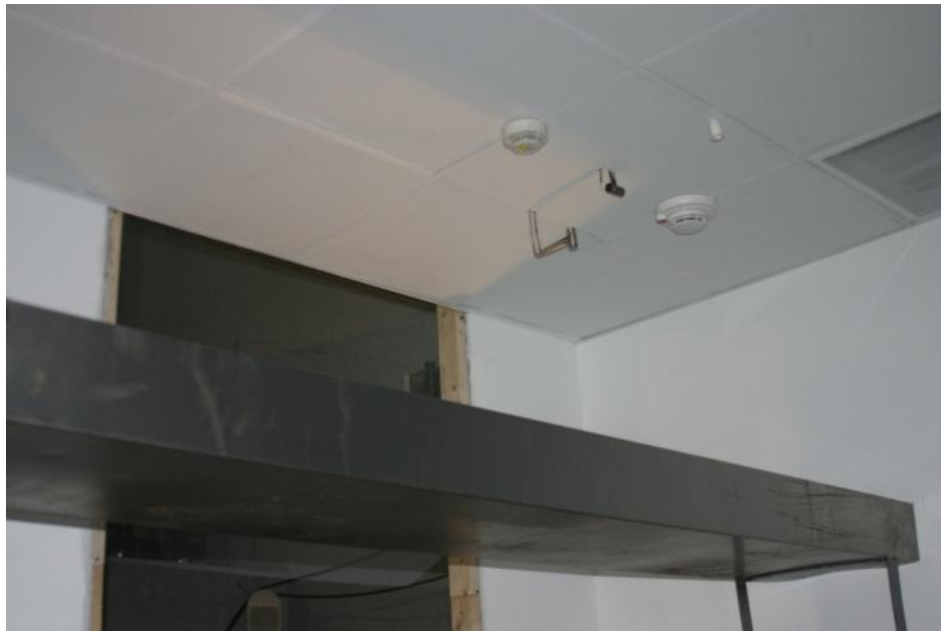
Figure 2-15: Picture showing the cable trays installed above the server cabinets.
