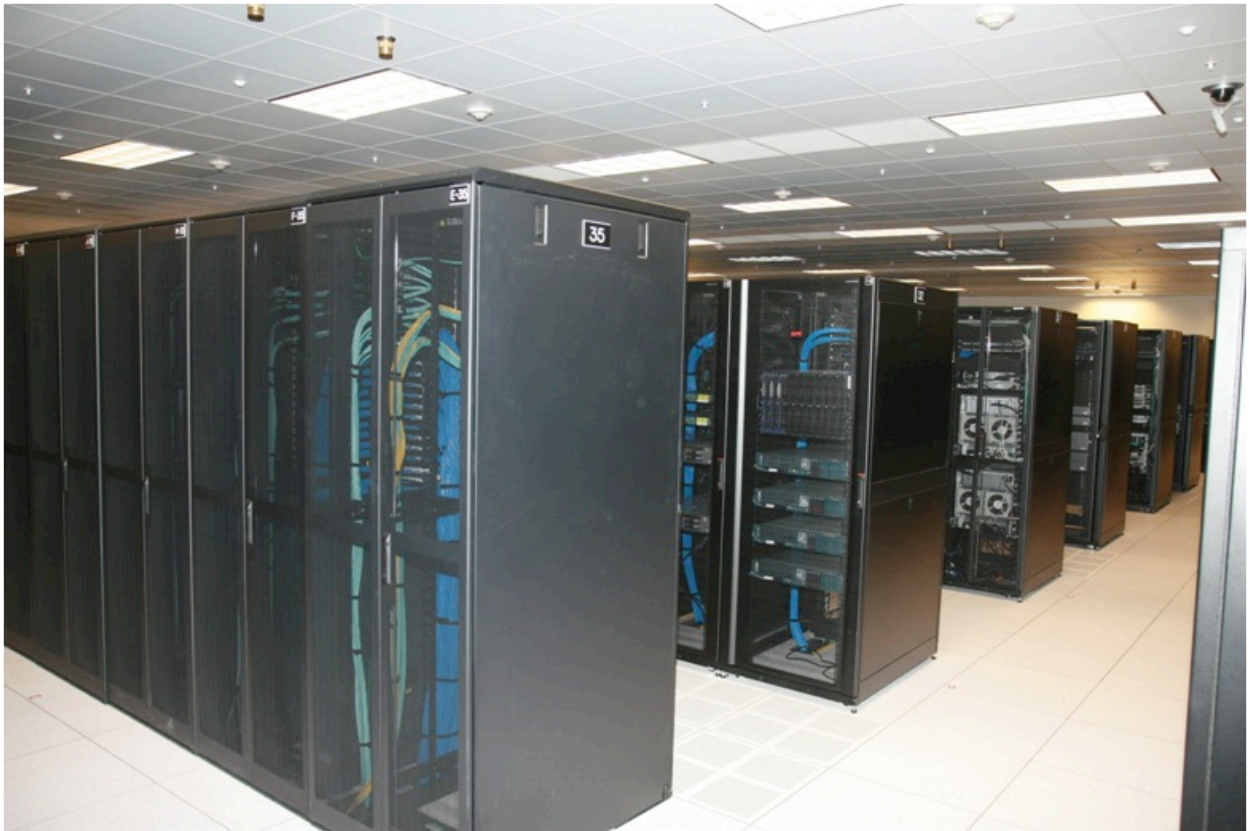
Figure 1-1: Sample pictures of a typical data center with arrangements of server cabinets.
