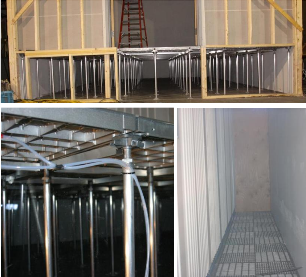
Figure 2-10: Photograph of the raised-floor during enclosure construction (top), close-up of floor panel support rods and underside floor grates (bottom-left), and top view of floor grates in the cold aisle (bottom-right).
