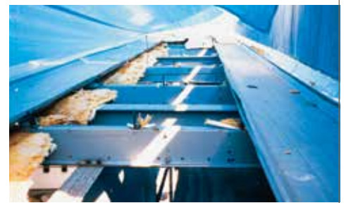
Panels of this standing-seam deck were torn off; leaving the fasteners still attached to the roof framing.
