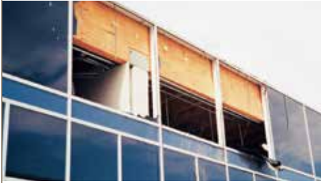
This glass wall facade was destroyed by high winds, leaving the building interior vulnerable to wind and rain damage.
