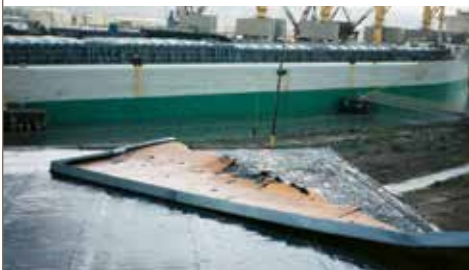
The damaged roof covering on this seaport building is mostly along the edge where wind forces are at a maximum.
