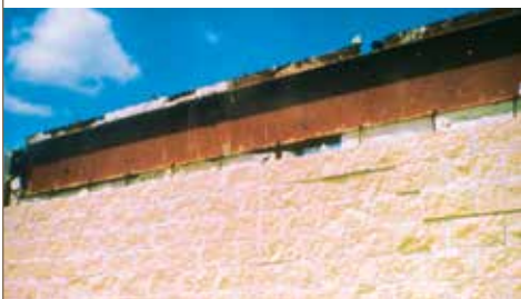
An inadequately designed parapet wall with masonry blocks was blown off at the roof line.
