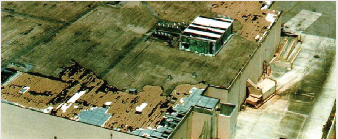
Hurricane damage to this roof is concentrated at the corners and perimeter, where the uplift pressure is higher.
