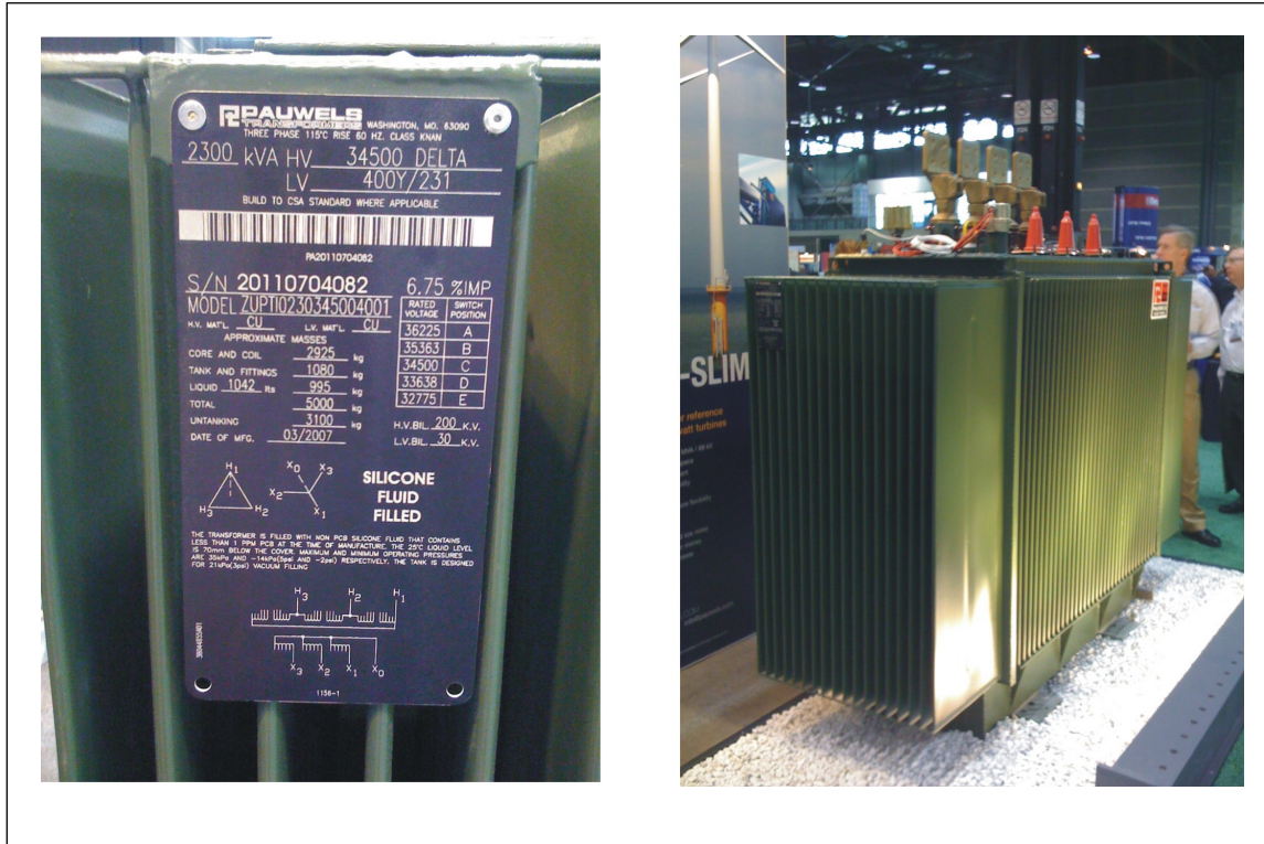
Fig. 3.4.4. A 2,300 kVA, 34.5kV/400V, Nomex insulated, silicon filled wind turbine generator transformer.
