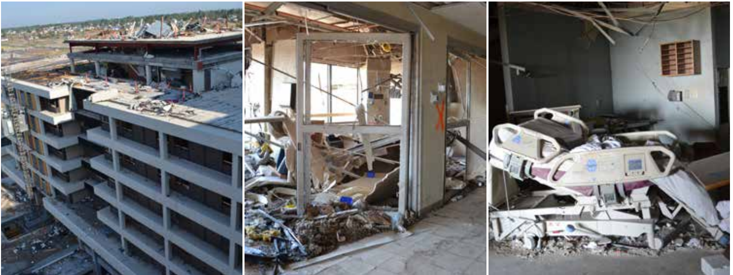
FIGURE 2: Devastating damage incurred at St. John's Regional Medical Center during the Joplin, Missouri tornado in 2011 [10].
